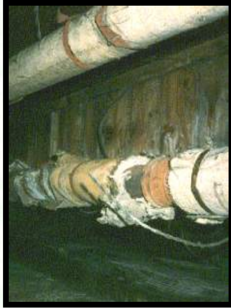
Asbestos insulated pipe in utility space
