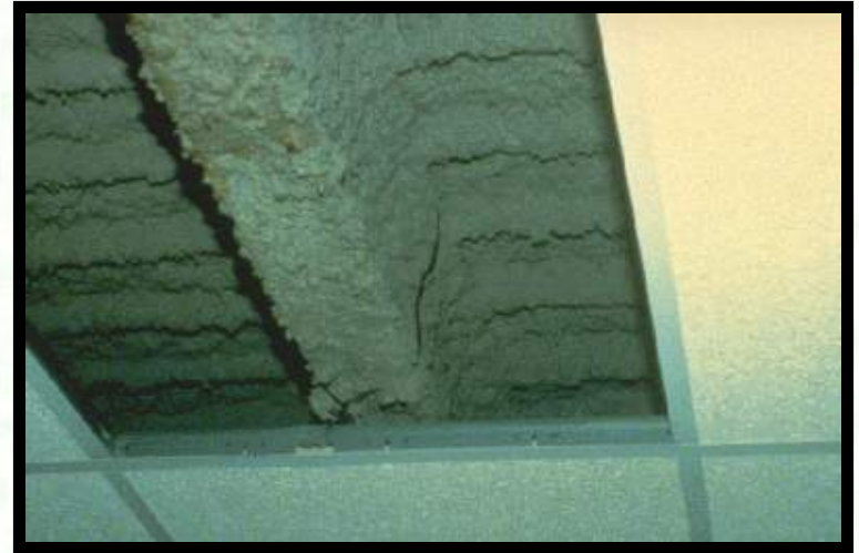
Spreayed-on fireproofing material
