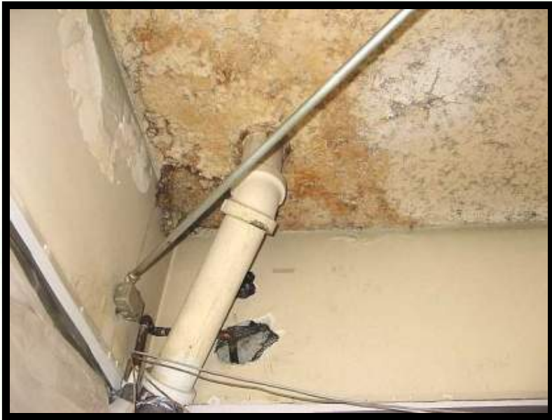
Water damage, deterioration
